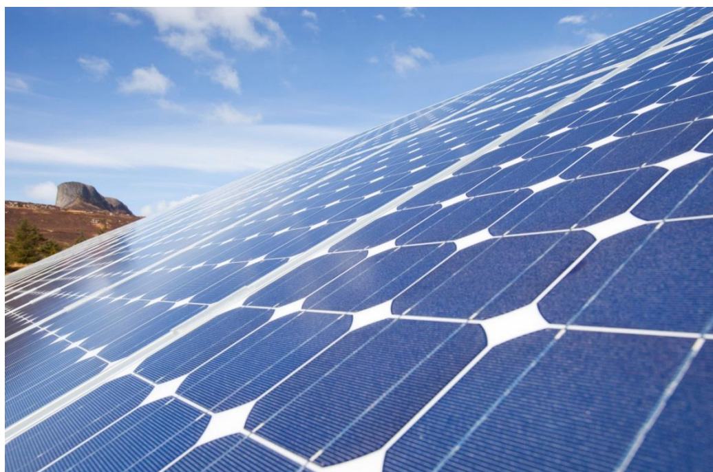
Arrays of solar PV panels on the Eigg off Scotland's west coast, UK. © Global Warming Images / WWF-Canon
